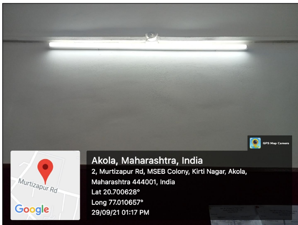
Use of LED lights
