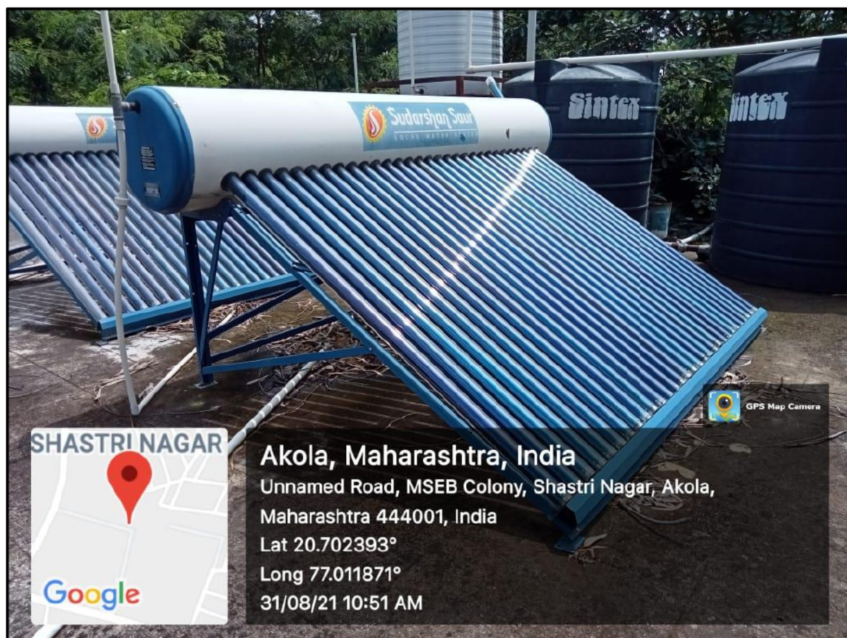
Solar Energy Point 1 & 2
